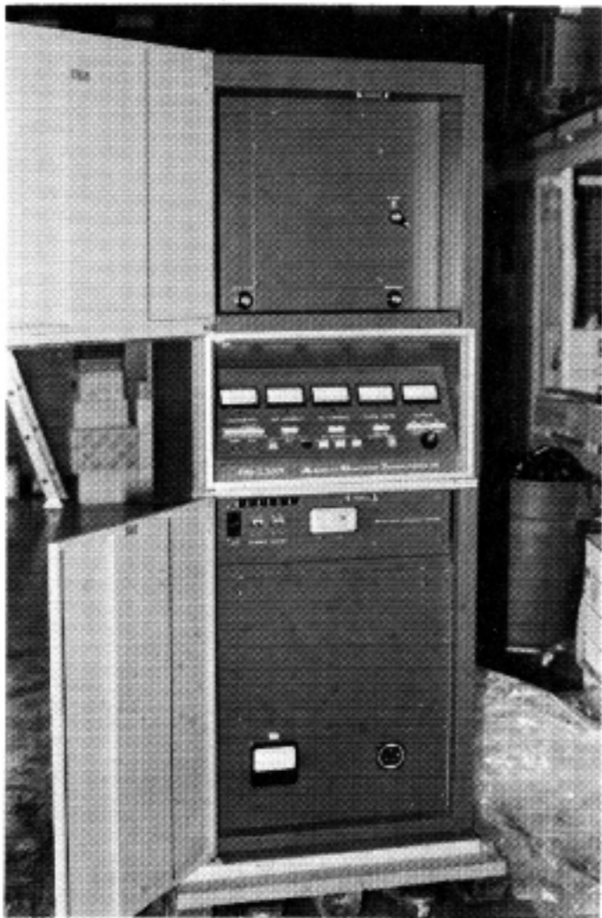
6X's 2.5 kw AEL transmitter is seen during installation. Station uses Optimod-FM audio processing.
