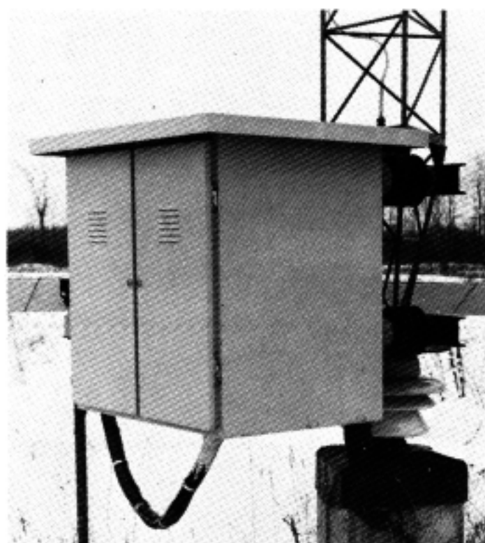
Aluminum cabinet at base of tower #1 holds antenna tuning unit with high voltage insulators visible at rear. In background is wooden trough carrying RF and power cable.
