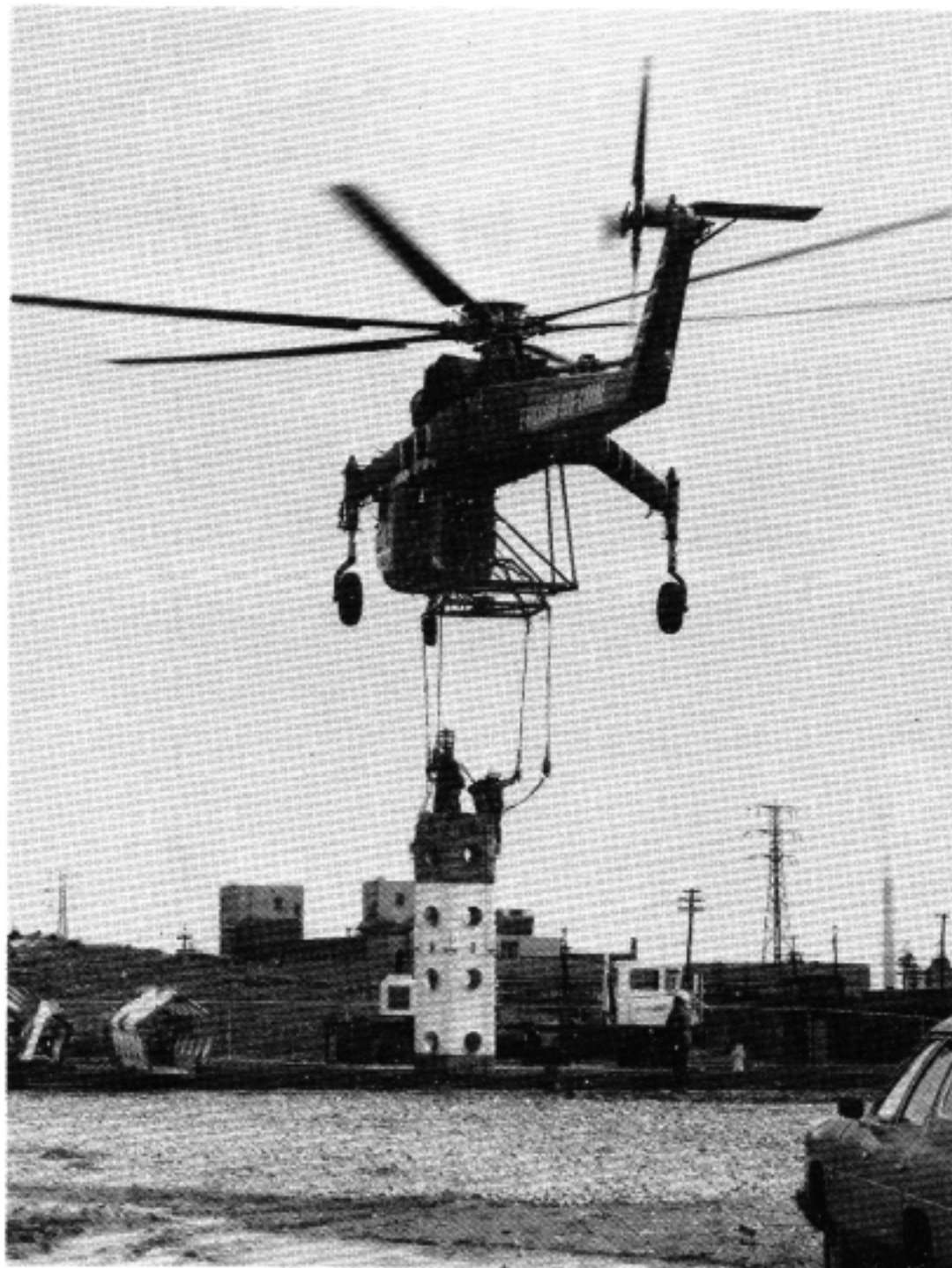
Down on the ground, workers attach choker cables to a section of the 335-foot antenna mast . . .
