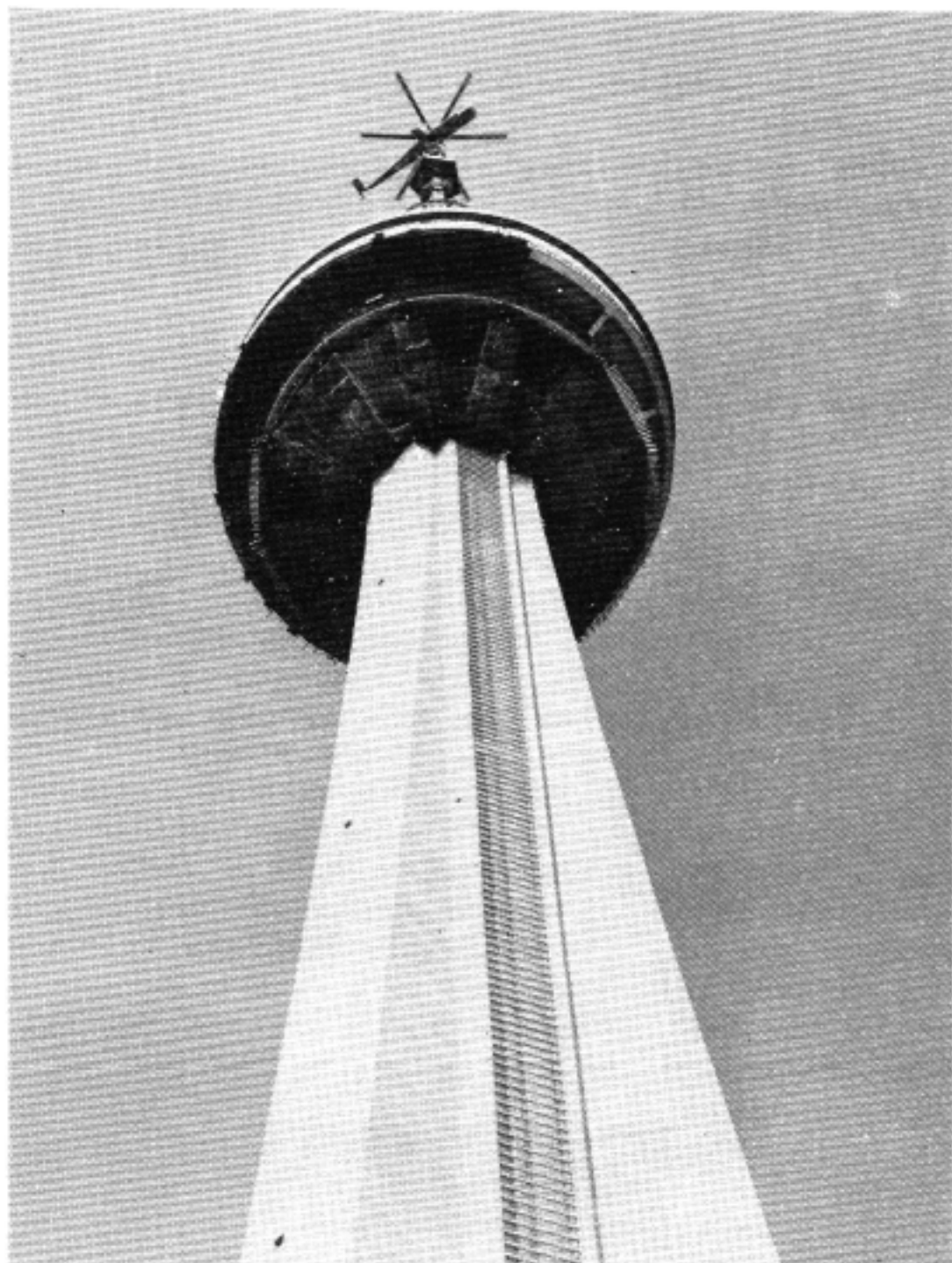
. . . the mast section is then whisked to the top of the tower and positioned by "Olga", the Sikorsky S-64E Skycrane.
