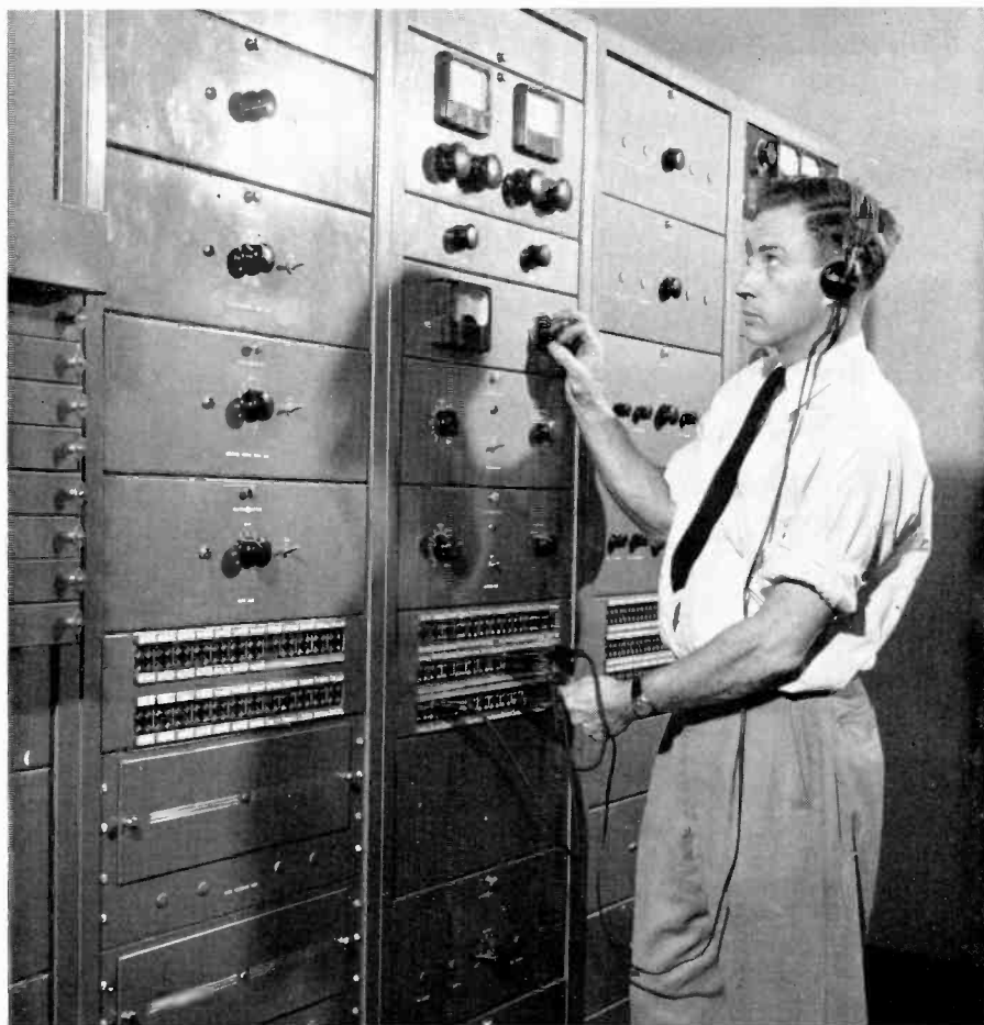
Figure 3.15B. Audio amplifier racks and patch panel in master control room at WRGB. Courtesy General Electric.
