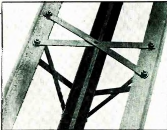
Fig. 6, below. This section carries three saddles to which the guy wires will be fastened
