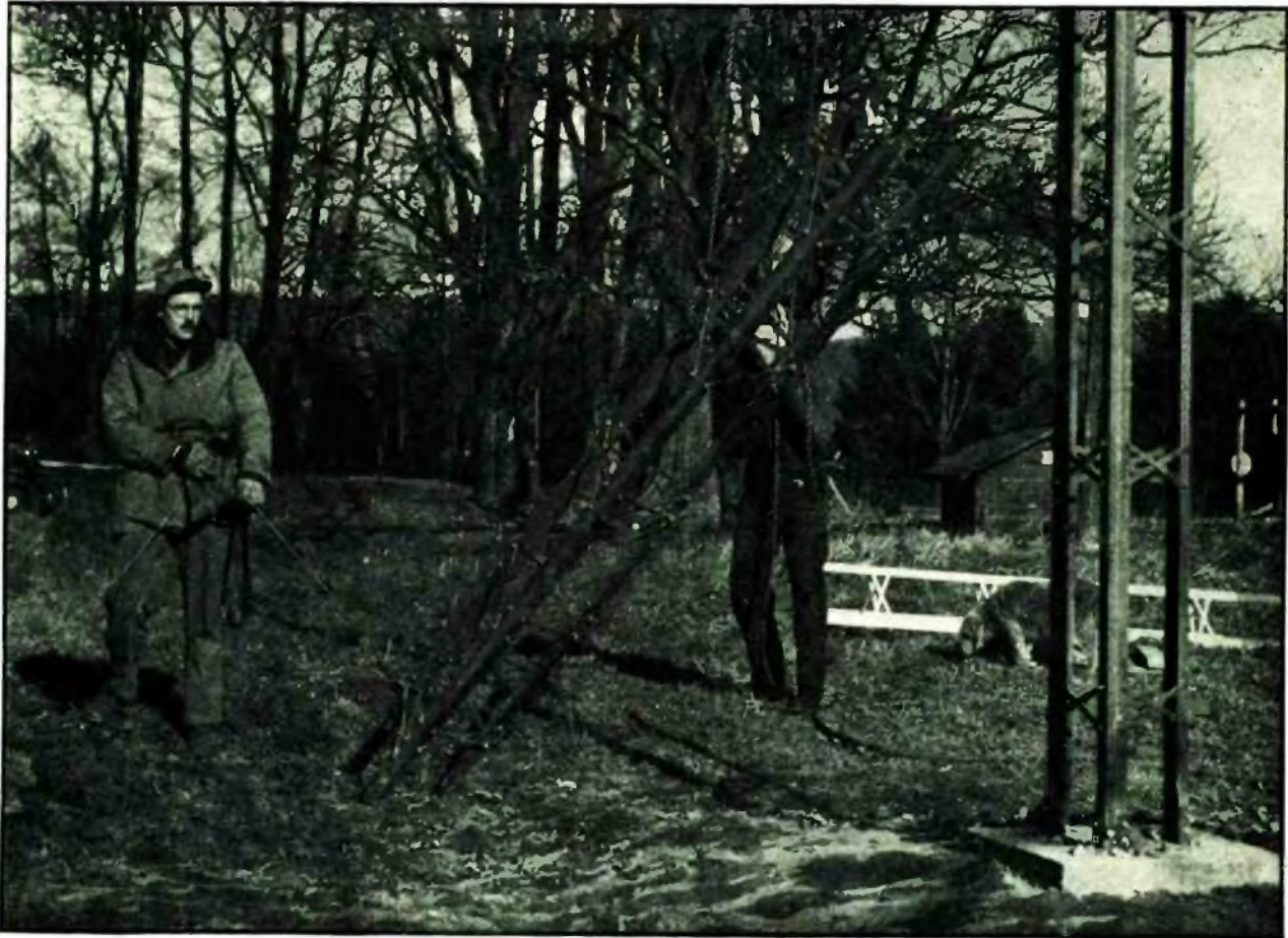
Fig. 1. Hoisting rope is attached just above middle of mast section. Small line steadies section on way up
