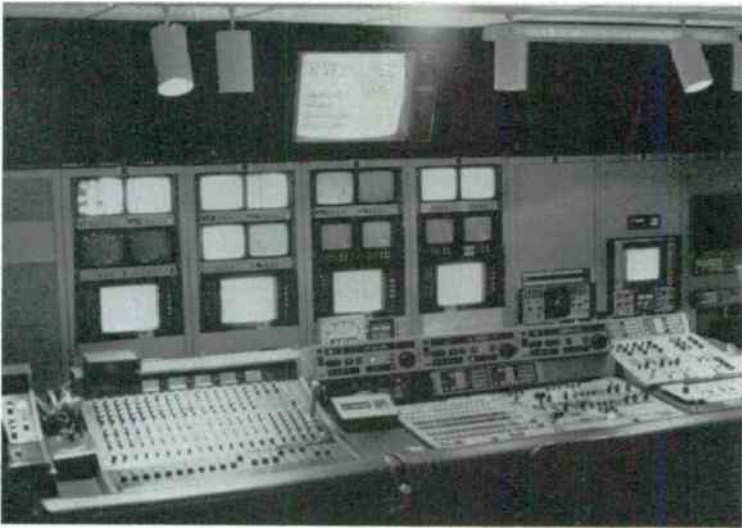
Fig. 10-2. The switching and monitor positions for the Eternal Word studios.
