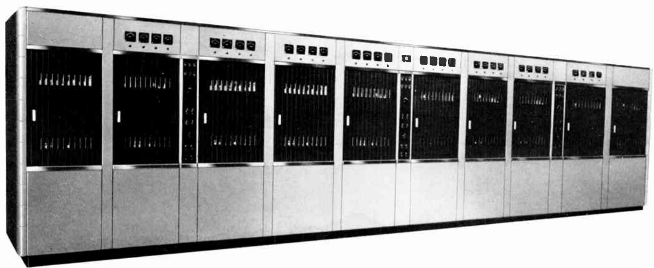
Below—Photo of cabinet line-up of the TT-25BL/BH Transmitter. In this photo rectifier cabinets are shown on the ends of the transmitter.
