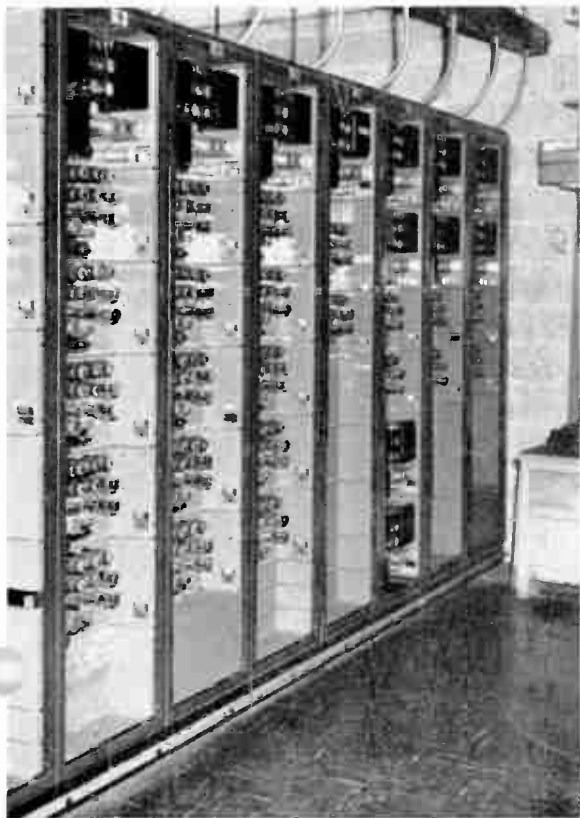
FIG. 39 (below). Fourth row of Master Control Racks which include the audio test equipment and additional power supply equipment.
