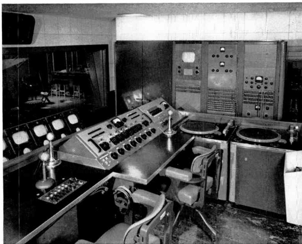
FIG. 22. View of a television studio control room showing video and audio monitoring facilities.
