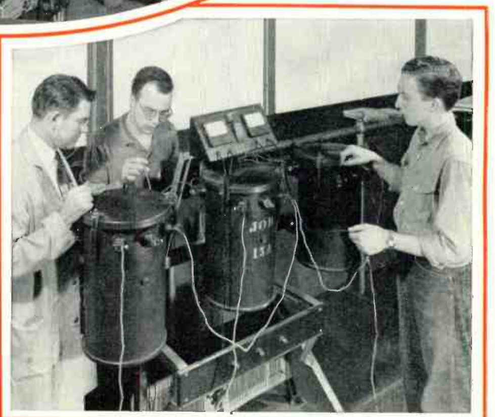
These students are connecting up a bank of power transformers for 3 phase operation, of a type commonly used in outdoor type substations.
