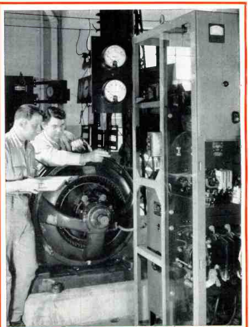
The above photo shows an Instructor explaining the operation and adjustments for synchronous type motor and students preparing to make tests. This unit is used for correcting Power Factor. Every trained maintenance man should be familiar with this type of work.
