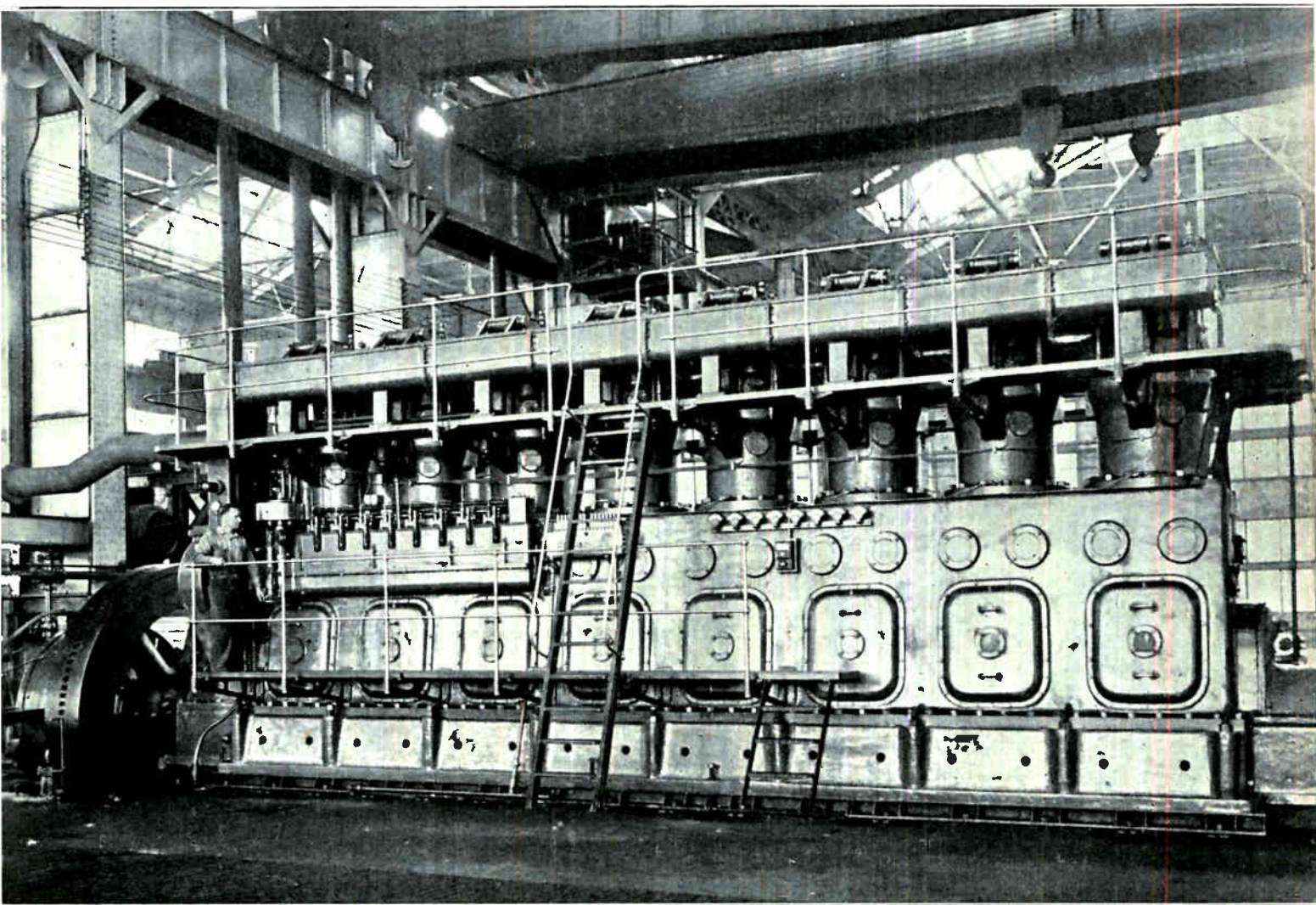
Fig. 63. The above photo shows a large heavy duty 200 RPM, 8 cylinder, 1600 h.p. Diesel engine. Note the operator standing near the control, governor, and fuel pump units. Also note the temperature indicating meters for each cylinder and the removable plates on the side of the engine frame to permit access to the bearings. (Courtesy Baldwin-Southwark Corp.)
