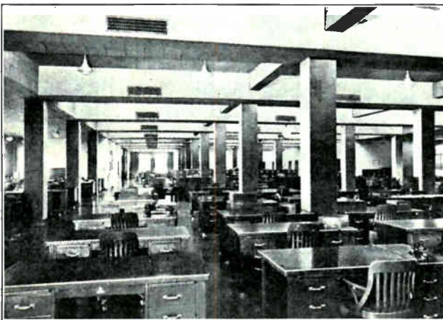
Fig. 148. Photo of the inside of a modern air-conditioned general office. Note the duct outlets along the ceiling beams. Much better efficiency and health can be maintained in such air-conditioned offices. Courtesy Jewell Tea Co.
