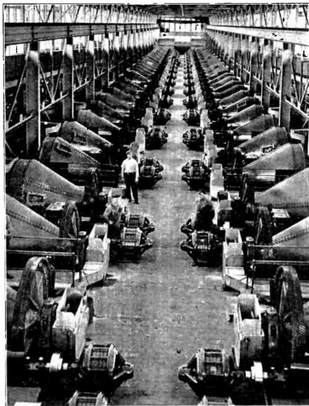
Fig. 475. This photo shows an installation of A. C. motors in a copper mill. Hundreds of thousands of motors in thousands of electrified factories and plants require the services of trained electrical maintenance men.
