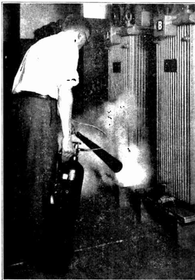
Fig. 474. This photo shows the use of a modern gas type fire extinguisher for fire protection in electric plants.
