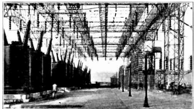
Fig. 414. View of large oil switches and lightning arresters underneath the bus and switching structure of a 220,000-volt outdoor substation. Courtesy of Philadelphia Electric Company.
