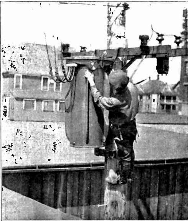
Fig. 124. This photo shows a pole type transformer and the method of making primary and secondary connections. Also note the thermotest temperature indicator near the hand of the electrician.
