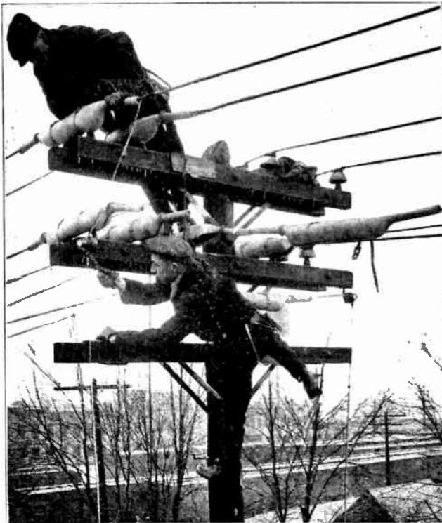
Fig. 368. This photograph shows the use of rubber line hose or "pigs" to protect linemen when working on live transmission or distribution lines. Photo Courtesy Lineman Protector Company.
