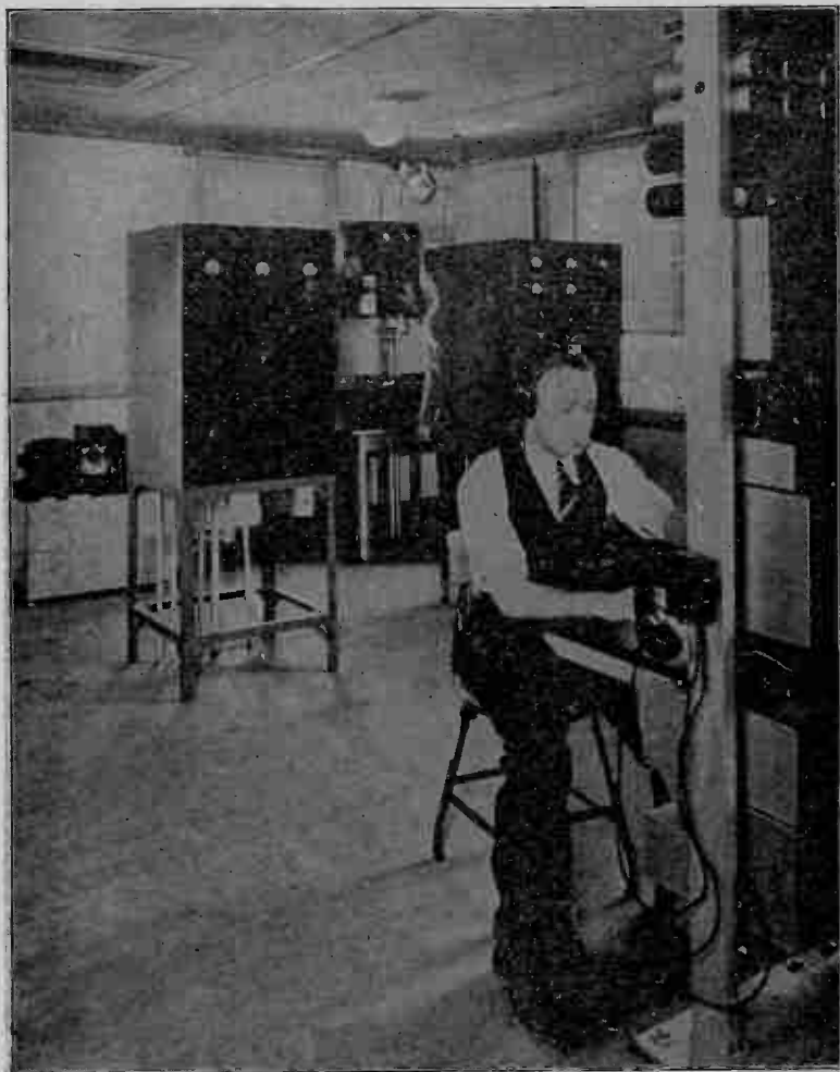
FIG. 5—Interior view of typical marine radio telephone station, (Courtesy Western Electric Co.)
