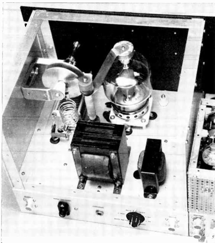
Fig. 17-6 — Interior of the 50-Mc. final amplifier. Plate tuning capacitor is modified neutralizing unit, left.
