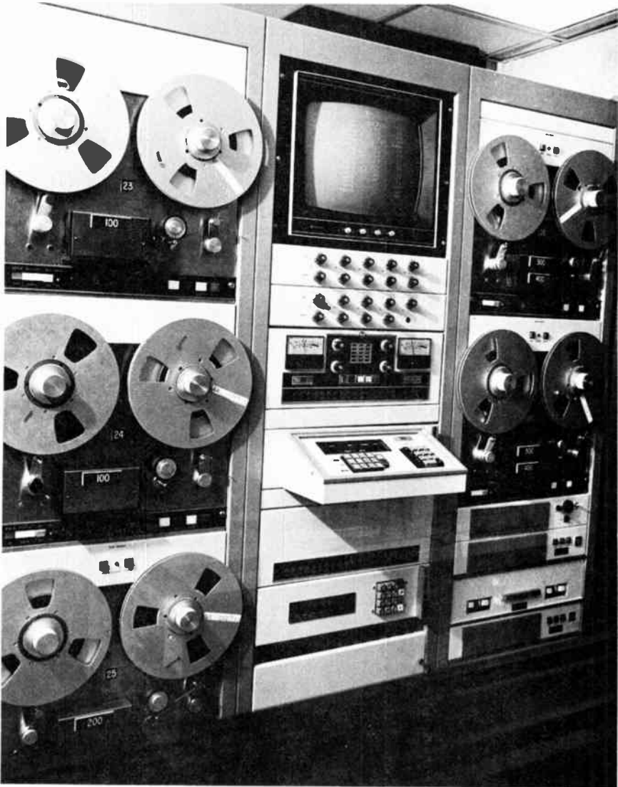
Figure 4.11 Control rack for Systems Marketing Corporation's DP-2 automation system in use at WBEN-FM, Buffalo, New York. The system has 40 channel switching, 8,000 programable events.
