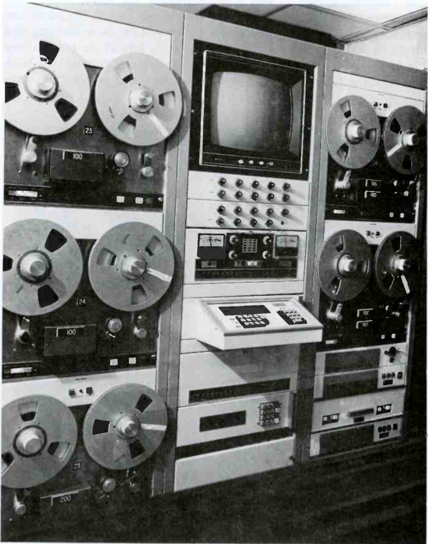
Figure 4.11 Control rack for Systems Marketing Corporation's DP-2 automation system in use at WBEN-FM, Buffalo, New York. The system has 40 channel switching, 8,000 programable events.
