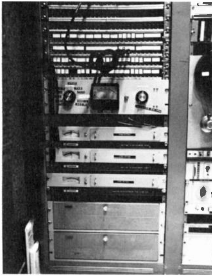
Figure 14.12. Equipment rack in a radio station.
