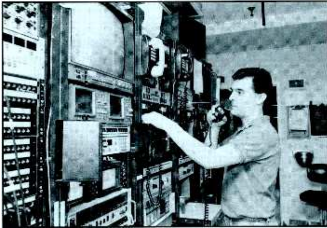
Taking in feeds from various sources is part of the duties of an Electronic News Gathering (ENG) crew.
