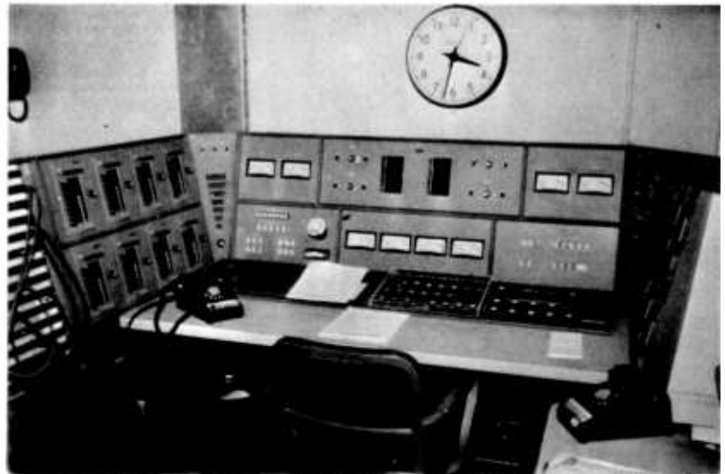
Fig. 16-3. ABC's transmission control console.
