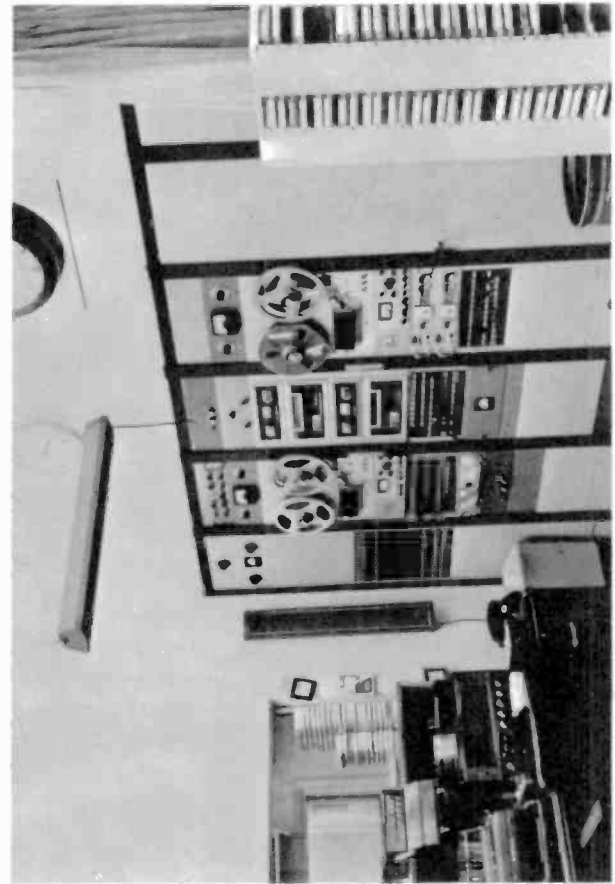
Fig. 16-15. Washington line recording racks in KYW's news gathering facilities.
