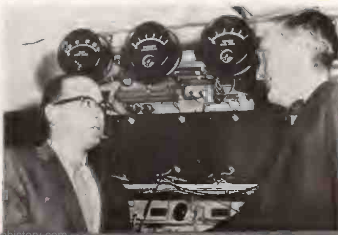
THANKS are given to Milton H. Klein (l.), general manager of KEWB Oakland, Calif., by Richard H. Baird of the Christian Broadcasting System. KEWB has donated the 1,000 watt transmitter shown to the religious broadcaster for use in Korean radio station.
