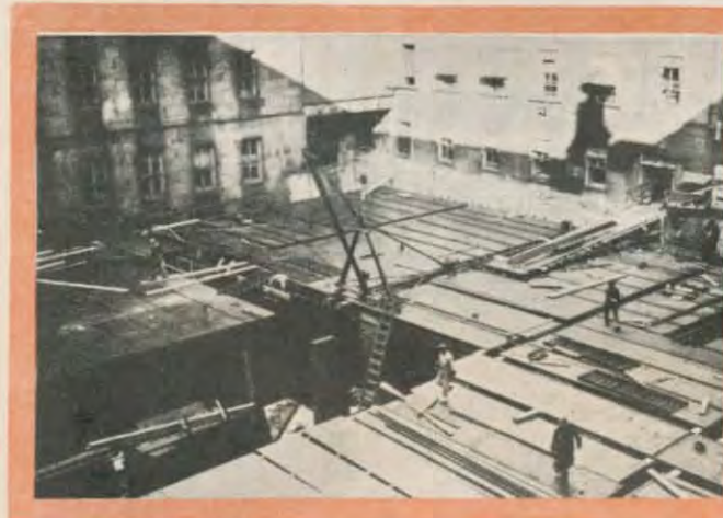
The new vault in course of building. It occupies an old courtyard of the Treasury building.
