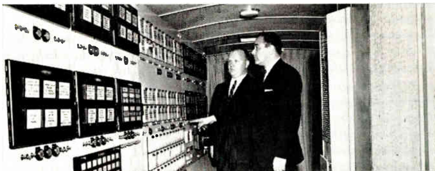
Fourteen-foot panel holding more than 20 different annunciators inspected by George Daniels, Jr., left, sales demonstrator, and George Mitchell, sales manager for the Scam Instrument Corp. Panel is mounted in a 26-foot bus now touring the U. S. for SCAM.
