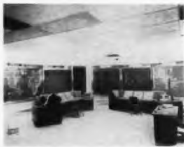
New Defense National Communications Control center is the "heart" of the Communications Control Complex. It will monitor and control the long-haul, non-tactical communications facilities of all services. Philco Corp. was prime contractor for the project.
