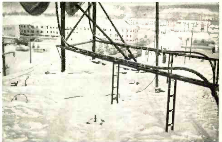
Styroflex cables connect transmitters directly to roof-supported dishes.
