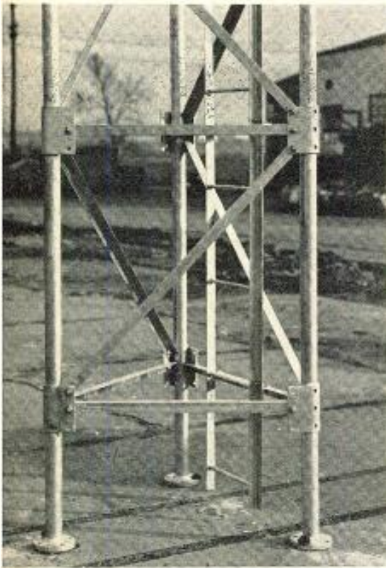
Part of triangular cross-section tower, showing flange steel wrap-around plate welded to pipe section, and angle iron bracing
