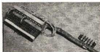
This method of terminating pairs on popular WE 100B block is found in many stations
