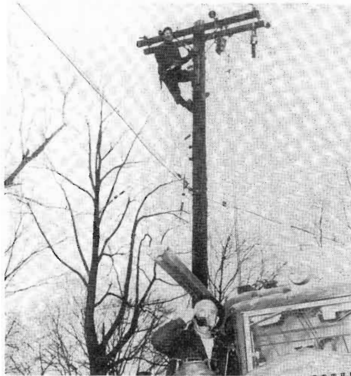
A crew foreman for the Niagara-Mohawk Power Corporation at Syracuse, N. Y., uses GE two-way radio in his repair truck to call for additional materials. Two-way radio helped speed up extensive repair work made necessary by recent ice and wind storms in the Central New York area.
