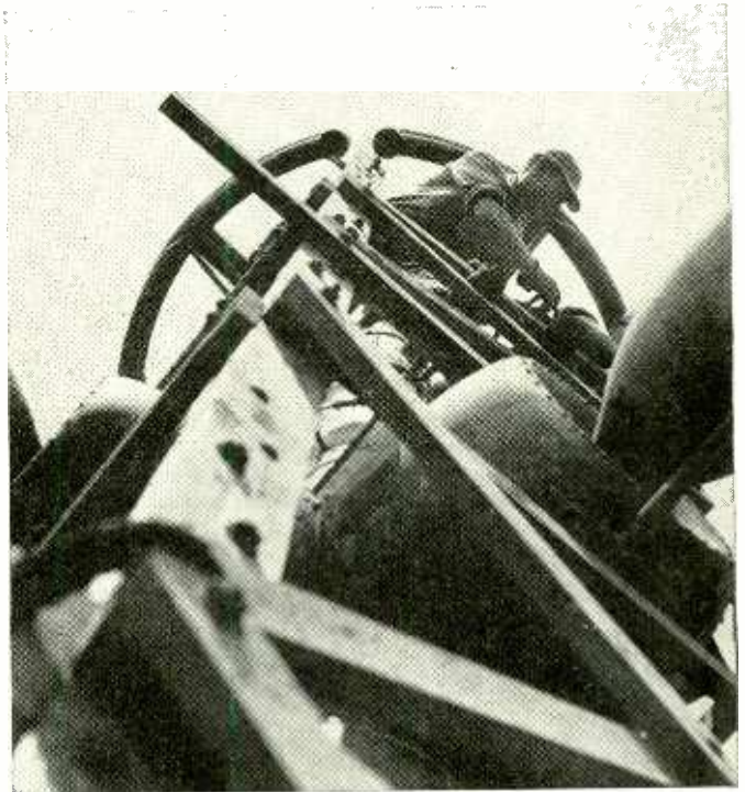
Steeplejacks at work on an NBC television antenna—1250 feet above the sidewalks of New York. Its height gives telecasts a wider range in the New York and New Jersey area.
