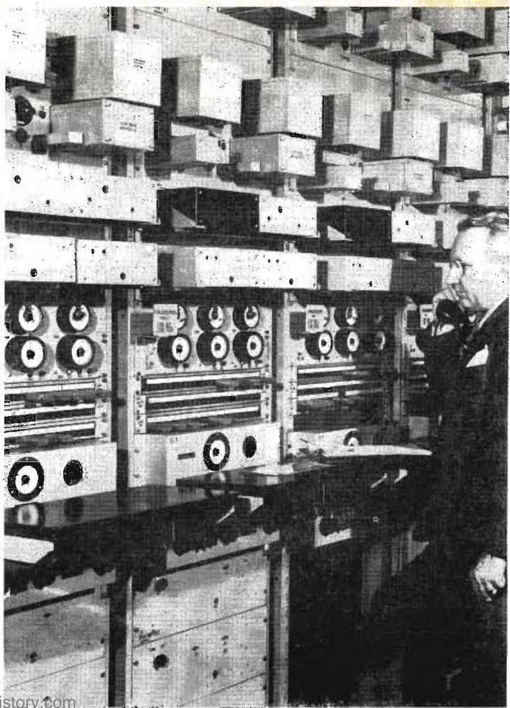
Cable terminating equipment contains amplifiers, regulators and equalizers. Dial pilot indicators show frequency levels in lines
