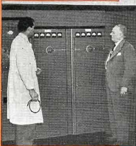
TWO FEDERAL 250-WATT TRANSMITTERS assure 24-hour service. One is in continuous service—the other stands by in case of emergency. Sgt. J. A. Stoltenberg, Police Radio Engineer (left) and Police Commissioner Hamilton R. Atkinson.
