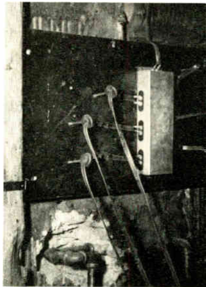
Fig. 3.—Distribution box located in the plumbing shaft at the 15th floor level. Six lines go to rooms above and below this level
