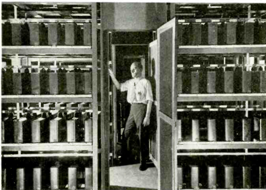
Bank of capacitors used to bring the power factor of the magnet energizing circuit up to unity. About 1,000 amperes are supplied and the resonant voltage is 4,000. Coils dissipate 120 kw
