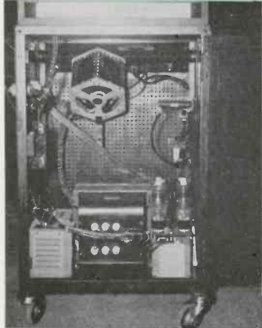
Fig. 3—Rear of power supply with interlocked protecting door open. 866 rectifiers at right
