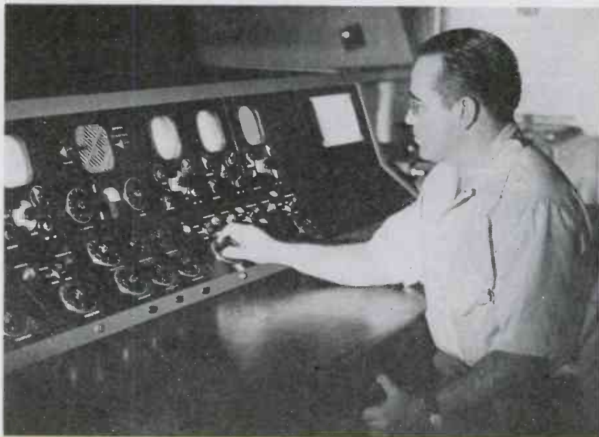
A complete system of modulation monitoring by means of oscilloscopes, and of frequency monitoring by secondary standard and WWV comparison is centrally located in the control room
