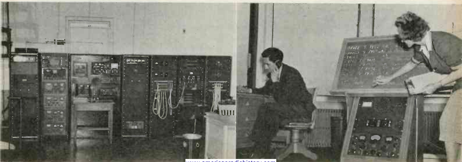
TRANSMITTER ROOM with low power, low frequency rig, monitor speakers, emergency equipment, high power transmitter and patch panel. Right, frequency meters
