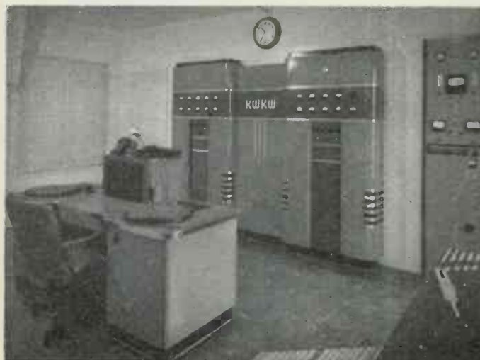
CONTROL ROOM and 1 kw transmitter
