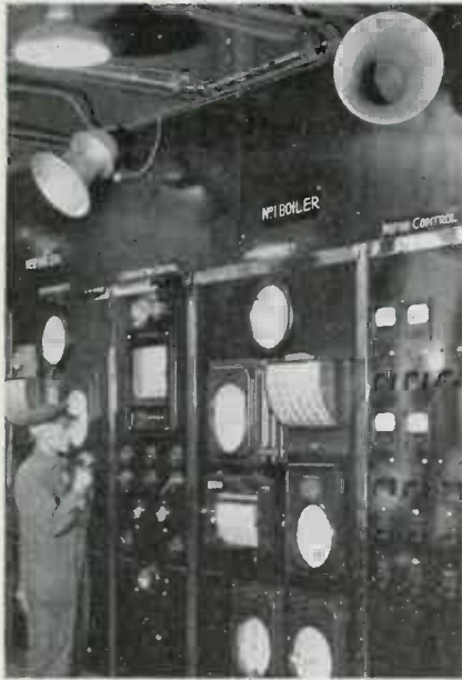
From boiler - firing level, operator can ask pump floor for more feed water and obtain immediate response
