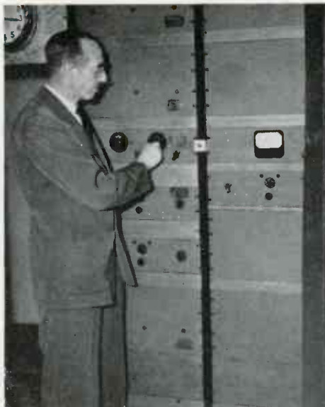
Chief Engineer O. B. Hanson at the controls of NBC's new clock system
