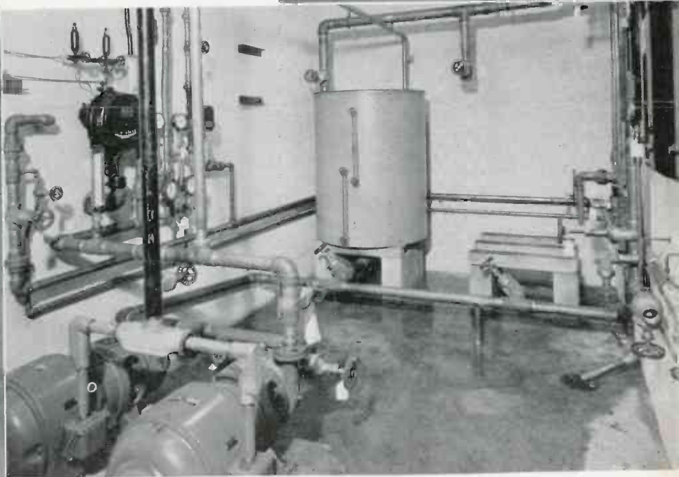
↑ Pump room in the basement. Picture shows the water-cooling equipment for some of the larger tubes on floor above
