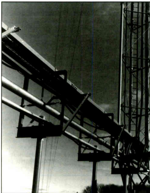
Andrew H-R line along the WGTU tower in Traverse City, Mich.
