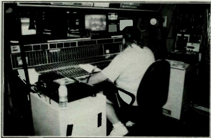
Both Control Rooms A and B featured Ward-Beck ST4842 audio mixing consoles.
