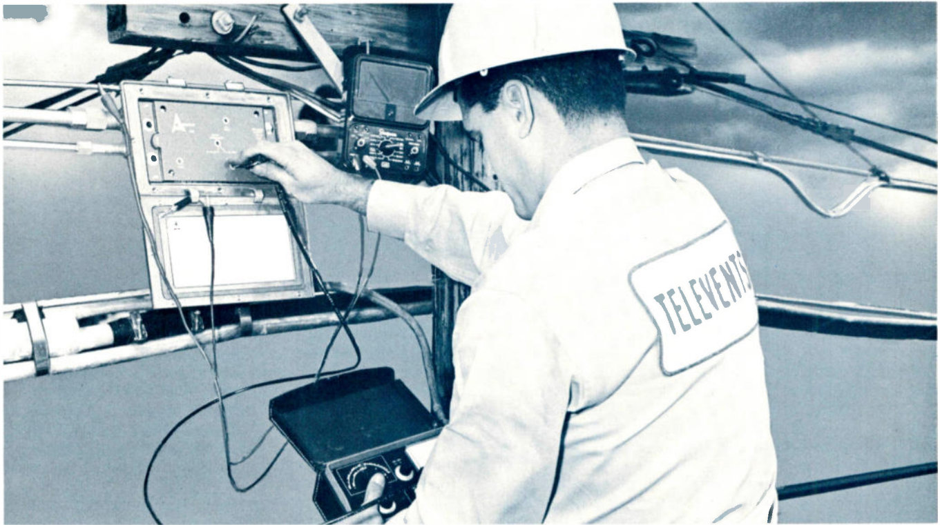
Televents of California Chief Technician Russ Salva installs AMECO PACESETTER in Pleasant Hills system.
