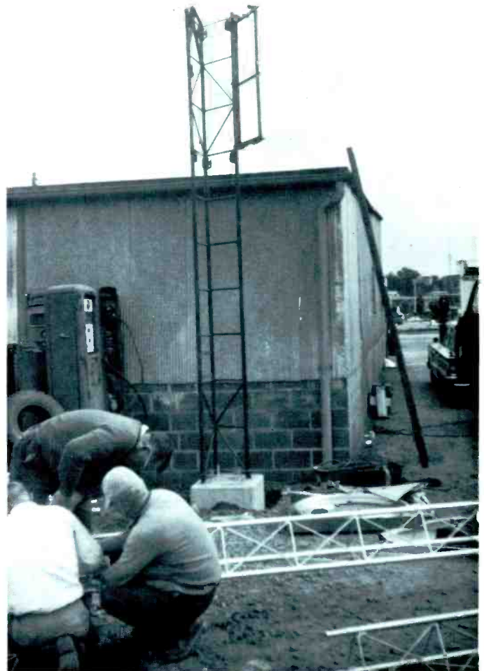
Kwik-Up Erector Kit installed on tower base and guyed, ready for first 30 feet of tower to be slid inside frame.
