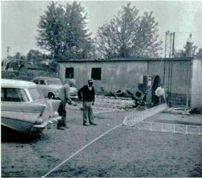
30 foot top section of tower and antenna erected and ready to be lifted into Kwik-Up Erector.
