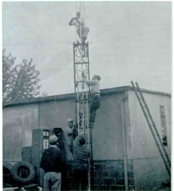
Guys are attached to section of tower already lifted above ground before the next section is cranked into place. This is as far as a man ever gets off the ground.
