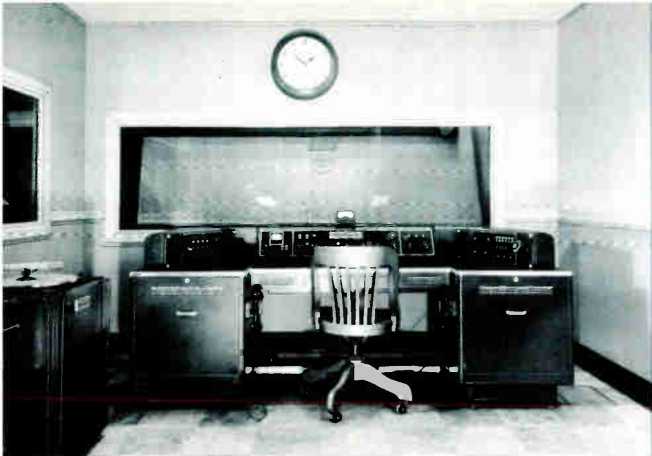
All WTMJ programs clear through this sub-master control room. Station WMFM has similar equipment in Radio City.
