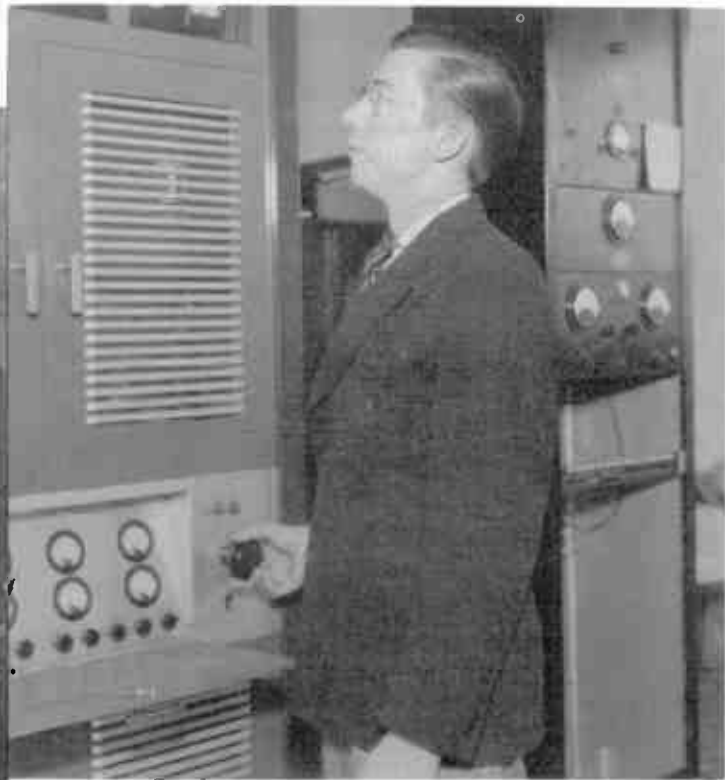
Operator WILLIAM ALFORD checking the meters that indicate the modulation and output of the WSJS transmitter.
