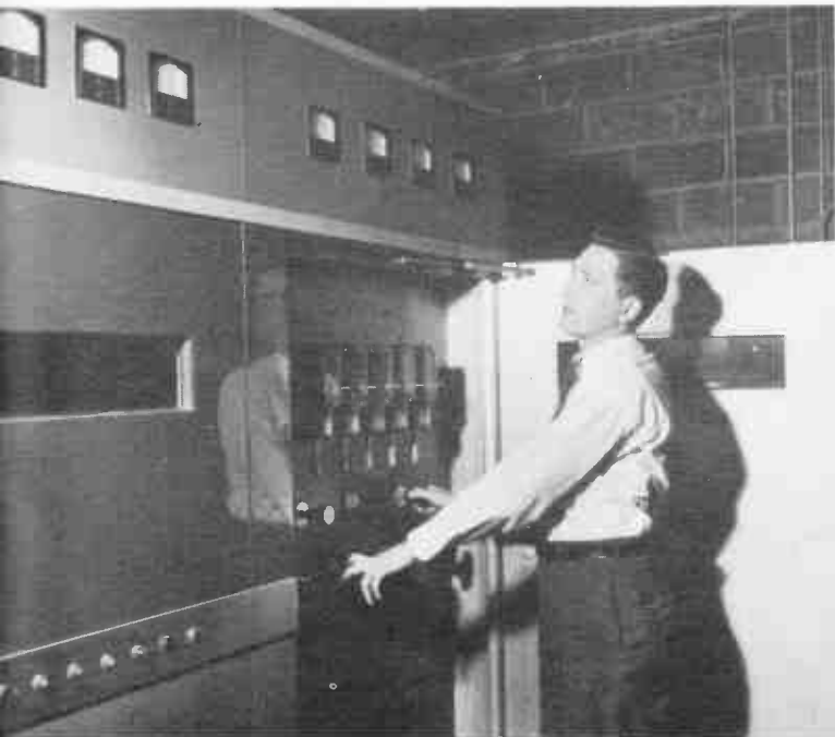
Frequent adjustments on the transmitter keep your favorite programs listenable. Here is Edward Grayden at the WREX 10,000 watt transmitter panel.
