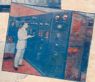
5,000 Watt Transmitter at Crete.
