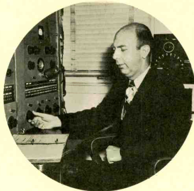
Al Osterhoff is in charge of the evening shift at the Transmitting Station for WKBB and WDBQ.
