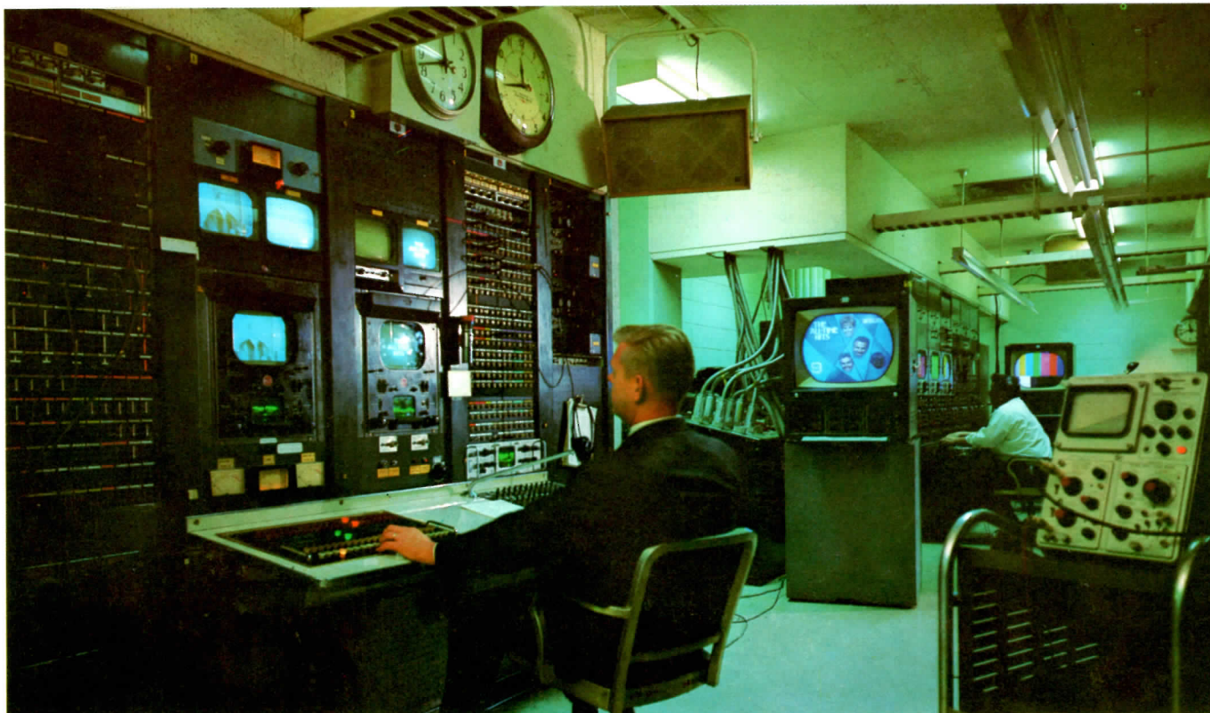
Television master control, where final audio and visual checks are made before transmission of picture and sound to the transmitter at the Prudential Building and ultimate antenna radiation.
