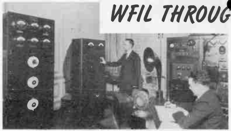
2 EARLY TRANSMITTER: The first WFI broadcasts came from the Strawbridge and Clothier Store . . . those of WLIT, from Lit Brothers. Together they became WFIL in 1935. ED DARLINGTON and DICK DELP were among WFI's first engineers. Both are with WFIL today.
