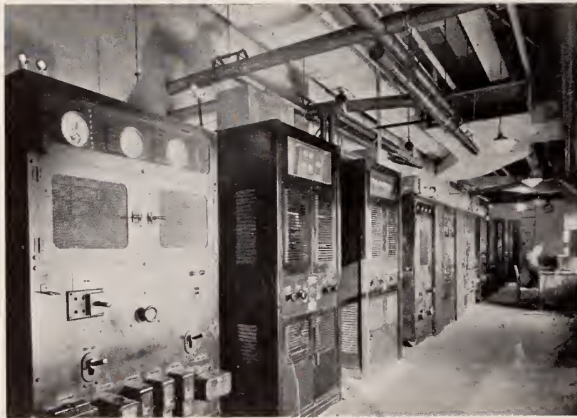
Empire State Transmitters—85th Floor
