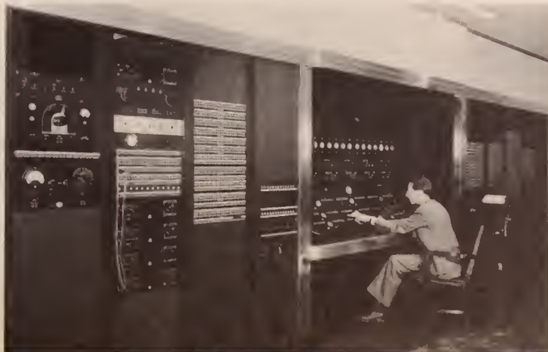
Below. NBC's Master Control Board in Cleveland with Engineer John Disbrow at the controls.
