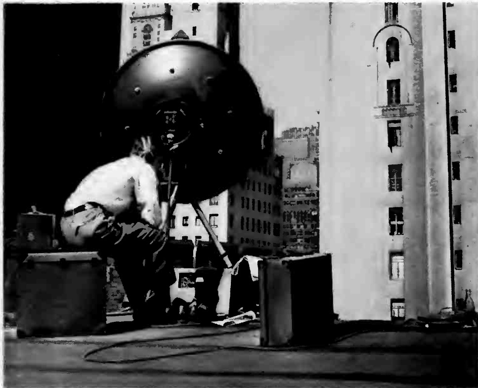
Parabolic transmitter, popularly called the "dish," reflects microwaves to the RCA Building in the distance.
