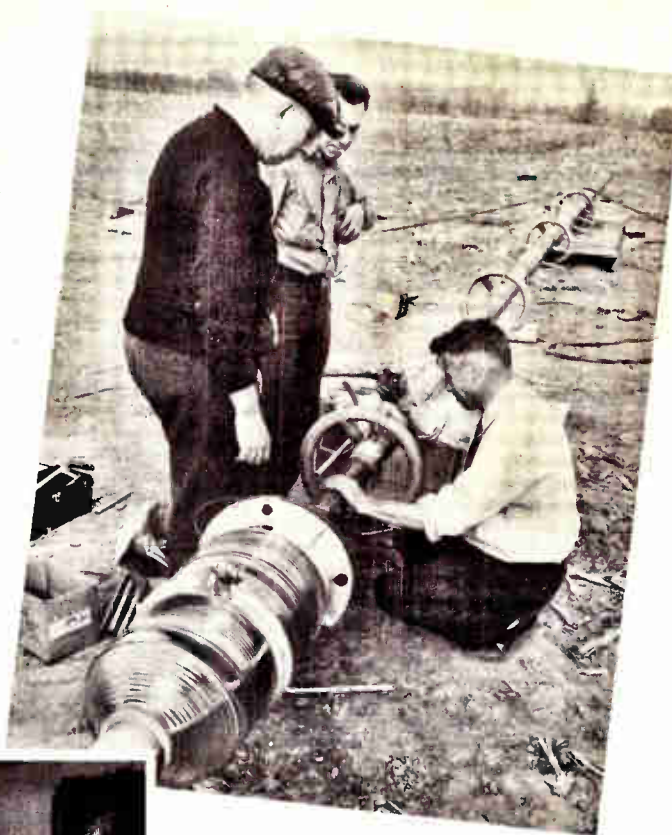
Engineers make final adjustments on the 4-bay FM antenna before it was hoisted to the top of the tall KFMX tower.
