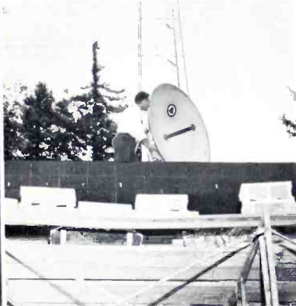
DISHPAN On roof of new television building, which is near tower (background), a "dishpan" antenna was also raised Thursday and was beamed to the dishpan tower on top of telephone building, where microwaves are sent.
