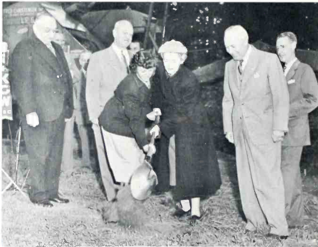
DIRT FLEW this morning at Council Crest park transmitter site of KPTV, city's first authorized television station. Hard ground drew heavy shovel work by Sandra Mayer (left), daughter of station owner, and Mayor Dorothy McCullough Lee. Amused spectators are (from left) City Commissioners Nate Boody and Fred L. Peterson. Edgar Smith, president of Portland Chamber of Commerce, and R. G. Freeman, vice president of Empire Coil company, holder of TV license.
